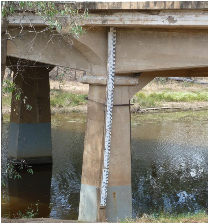
Fig A1-4 Gauge on the Avoca River Upstream South side of the Charlton Bridge
