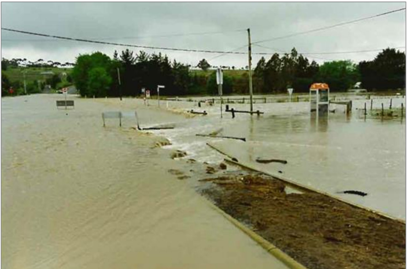
Figure 52. Flooding adjacent to the Midland Highway Bridge during the 1995 flood event.
