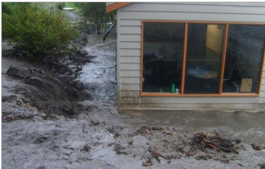
Parks Victoria office building flooded, January 2011 (Parks Victoria).
