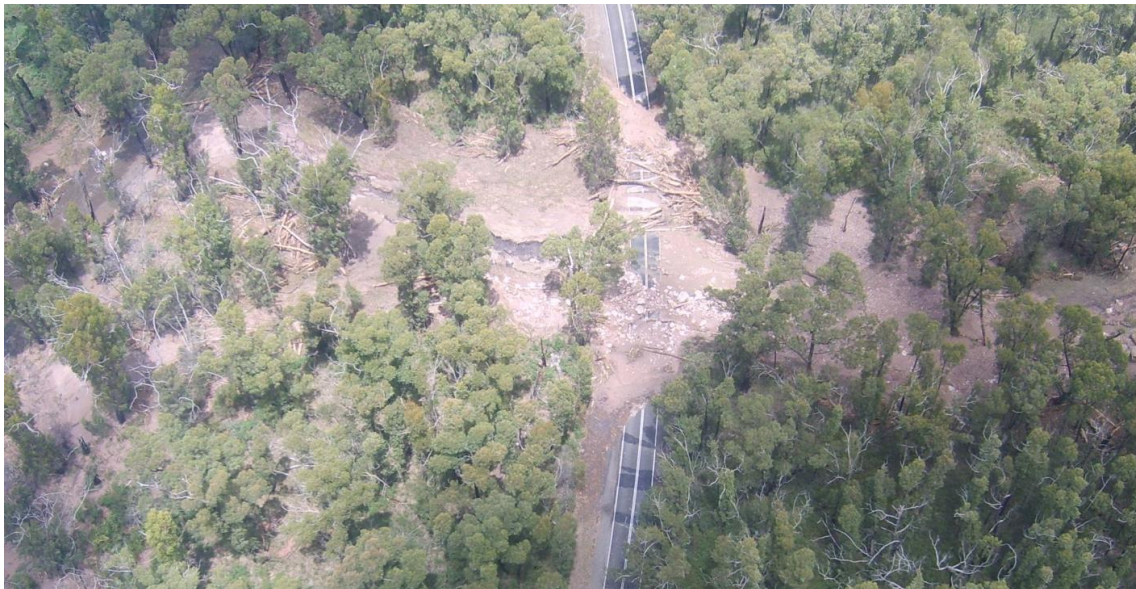
South of Halls Gap, access to Grampians Road was cut by a landslide, January 2011 (Parks Victoria).
